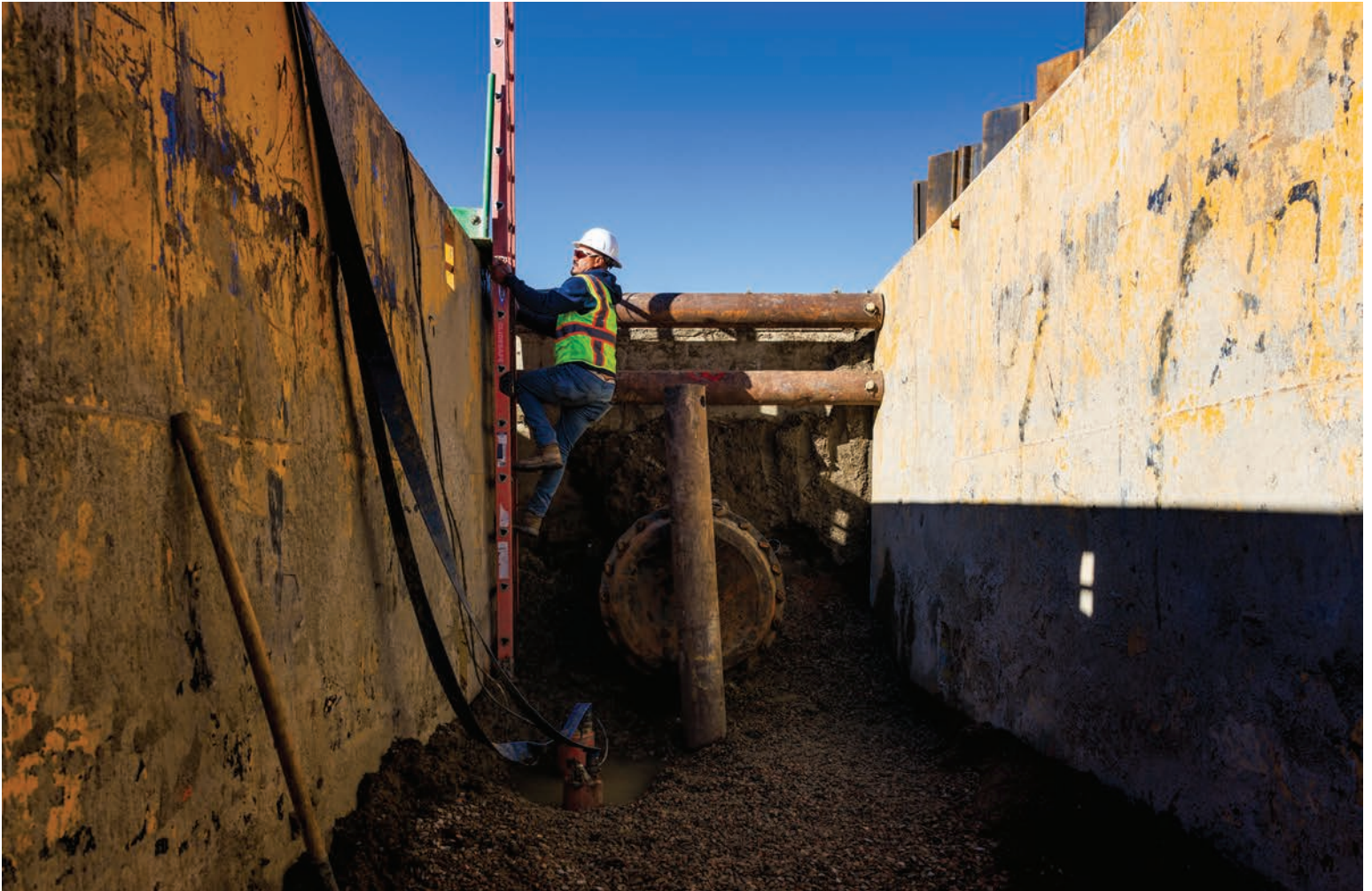
Orlando Rodriguez, Pate Construction foreman, climbs out of a hole where sections of the Arkansas Valley Conduit will be connected. Michael Ciaglo
