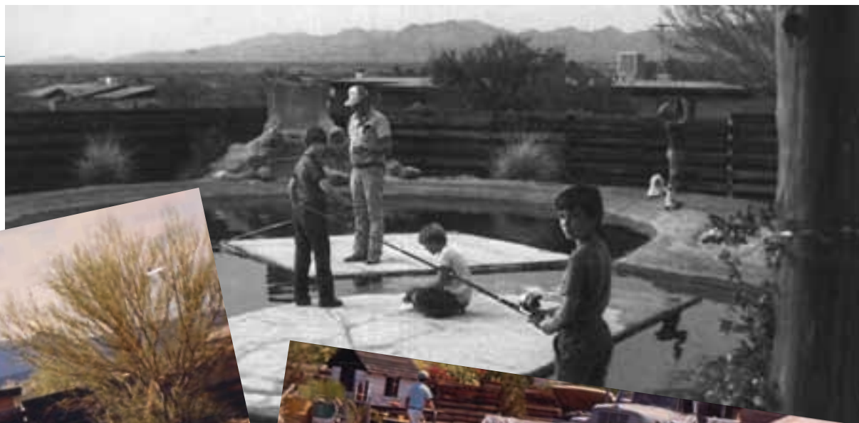
Clockwise from right: Cub Scouts fish in Brent Cluff's pond, catching some of the 200 rainbow trout Cluff had stocked from a northern Arizona fish farm. Workmen spray gunnite, the pond's basic raw material. Brent Cluff's daughter, Shawna, walks along a walkway separating two sections of the pond, still under construction. COURTESY CLUFF FAMILY
