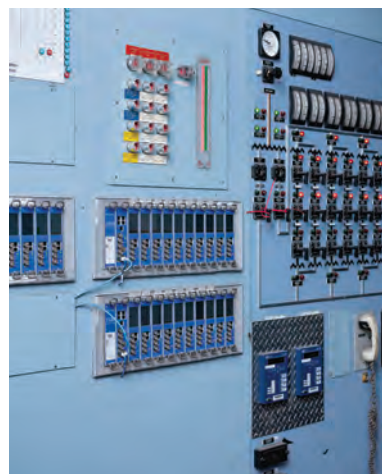
The control room of the Boardman Power Plant (left). High-voltage electrical transmission lines in Boardman, Oregon (right).
