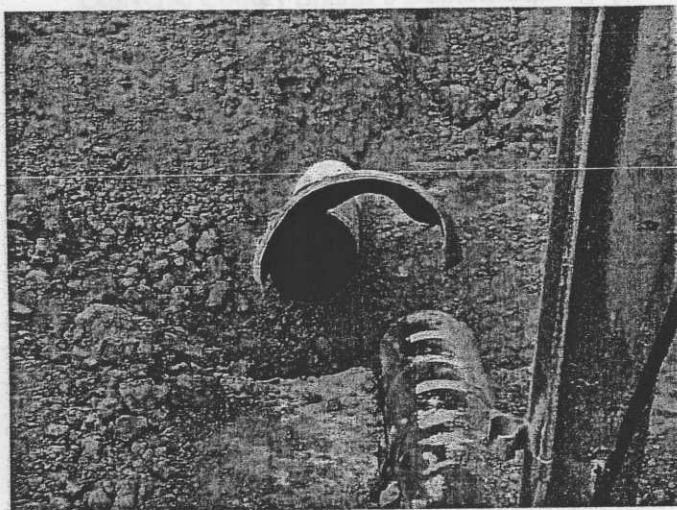
Photo #23 This photo shows the lateral misalignment of the ruptured pipe following the mishap. The sections of the 12" pipeline are offset by more than one pipe diameter.
