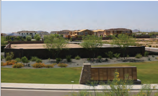
Construction underway at a new development in northeast Phoenix, purchased from the Arizona State Land Department. BROOKE WARREN
